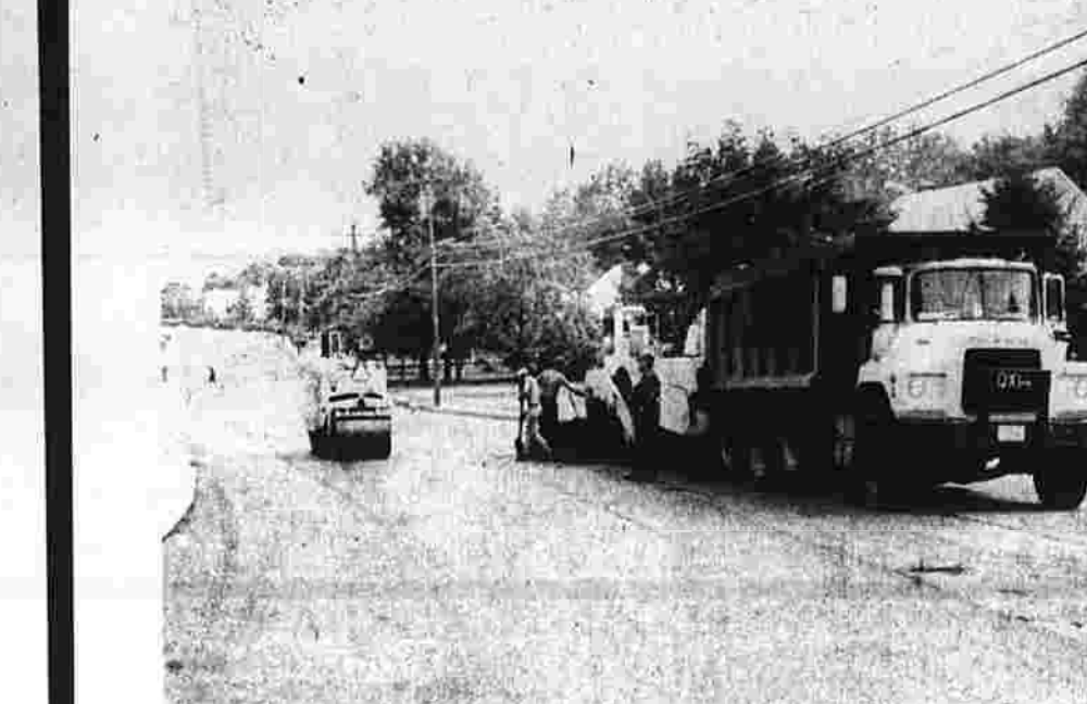
Repaving Road crews were busy Friday afternoon as they resurfaced a section of South Adams Street. (Herald photo by Pinto)
